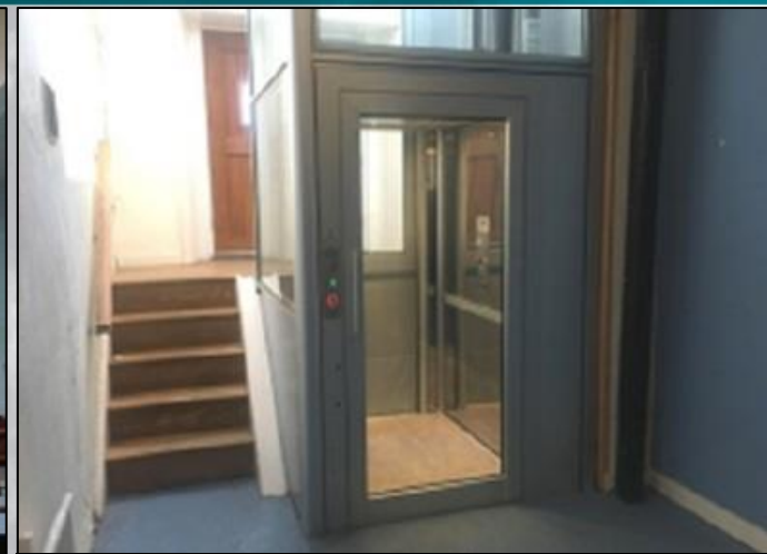
Platform Lift (Less than 6 years old)
